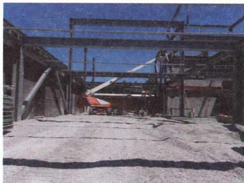
The previous main office space has been demolished to create a new main entrance and central commons.
